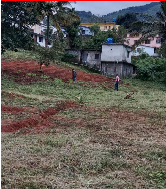
Fig: 3. Land has been affected by long longitudinal cracks and gully erosion
