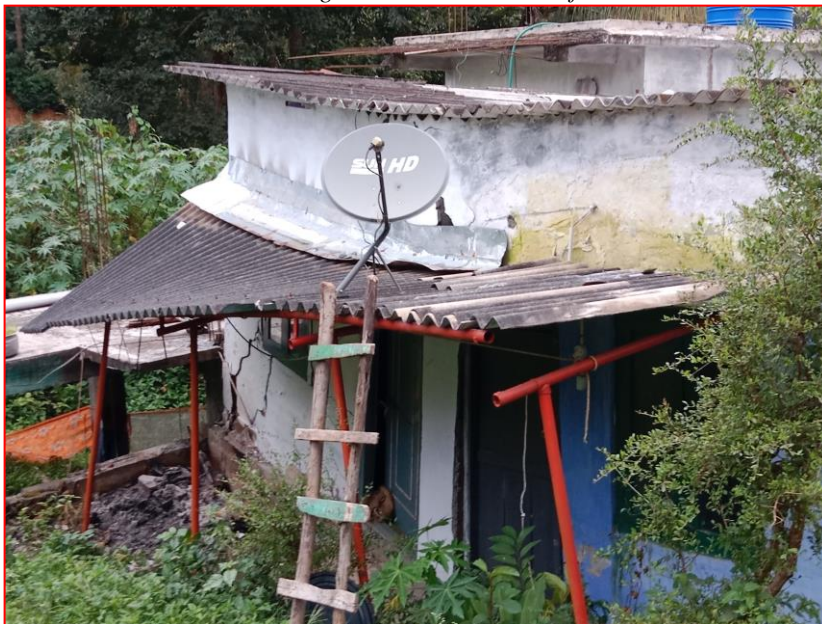
Fig.6: House got completely damaged due to subsidence and creeping
