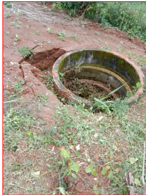
Fig.4: Well got submerged due to subsidence and creep
