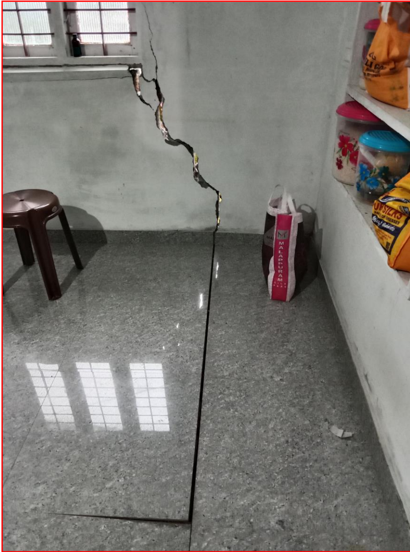
Fig.5: Crack in Wall and floor
